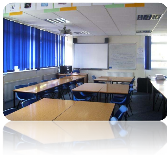
Figure 3.2 - Typical installation for a projector in a secondary school class
